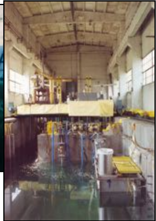
Spent fuel building (during canning team effort)
